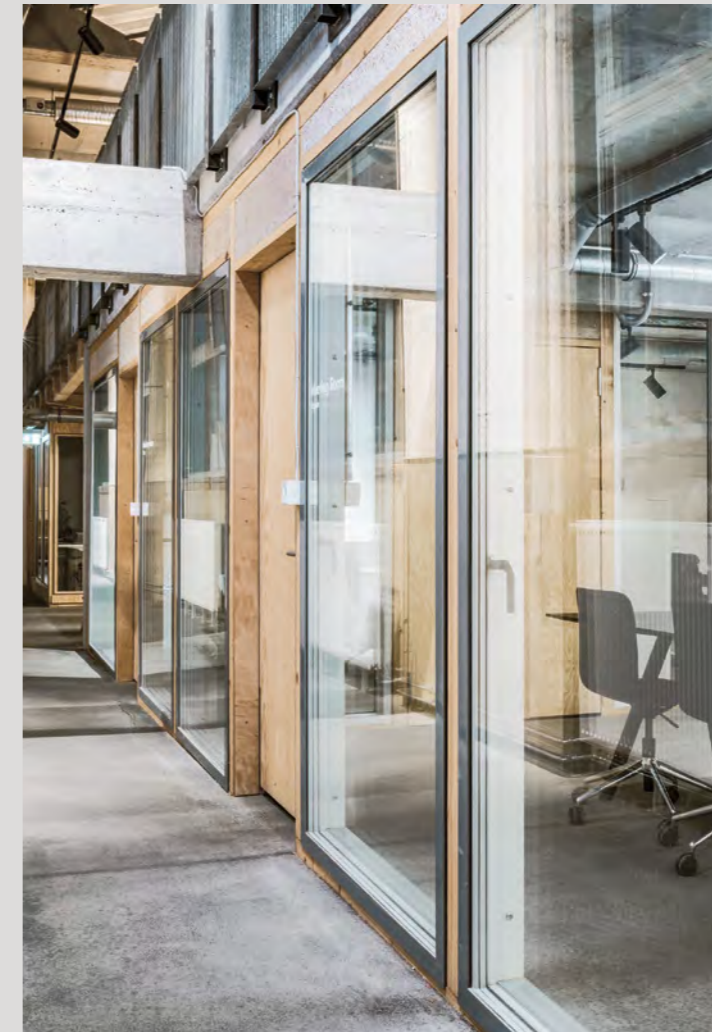
FIG. 12 Double-glazed windows are reused as partitions between the hallway and individual meeting rooms.
